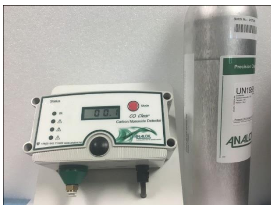
Connecting of the gas cylinder
