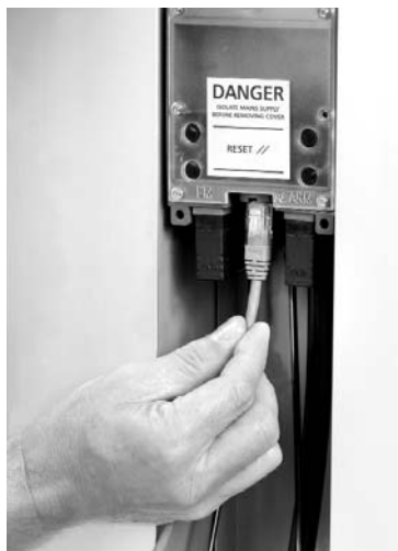
Connecting the PC to the controller
